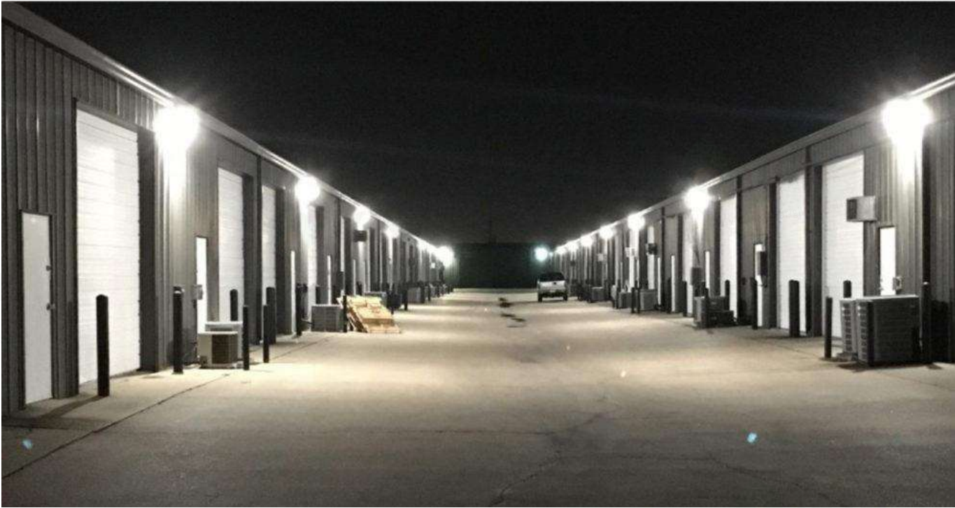
Figure 63. Wall pack lighting in warehouse exterior
