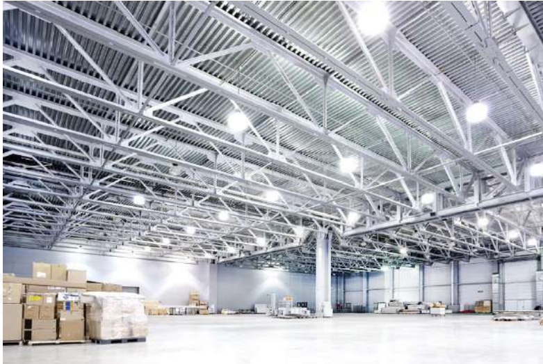
Figure 51. High bay lighting in a warehouse
