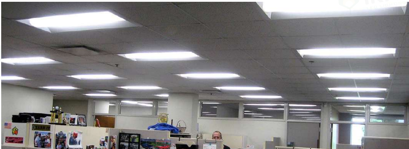
Figure 81. Troffers typically fit into a modular recessed ceiling grid
