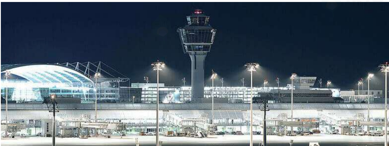
Figure 59. High mast lighting in an airport
